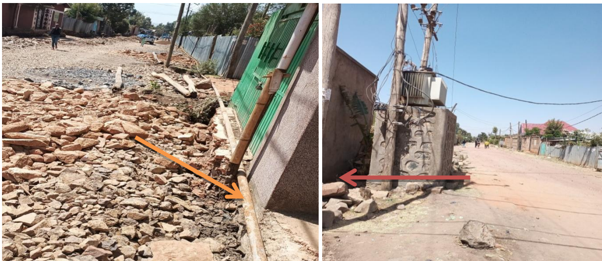
Figure 5 Utilities are not in place as per plan (Ambo), which can be obstacle to Traffic
